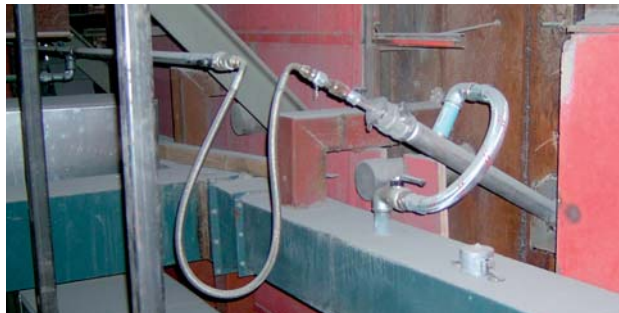
Water injection nozzles mounted through boiler casing and brick wall. Nozzle is cooled with compressed air.
